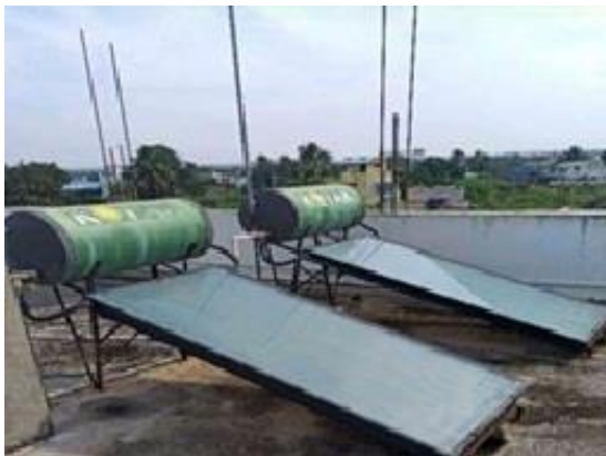
Solar Water Heater
