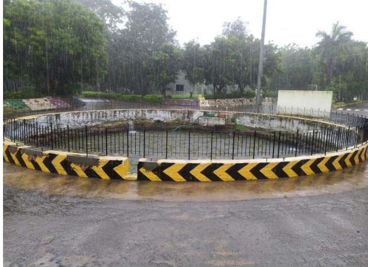
Rain water Harvesting Pond (4250m 3 )
